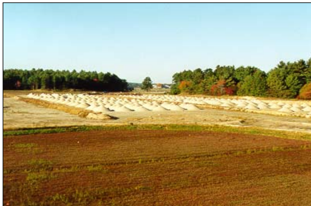
Figure 3. The mounds of sand represent the area where cranberry beds are being installed. These beds also represent an area formerly mapped as Hinckley soils. The bed in the foreground is a traditional cranberry bog containing peat (Swansea soil series).
